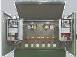
PAD MOUNTED SWITCHGEAR
